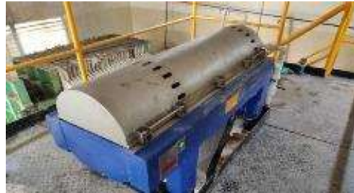
Decanter for Sludge Handling
